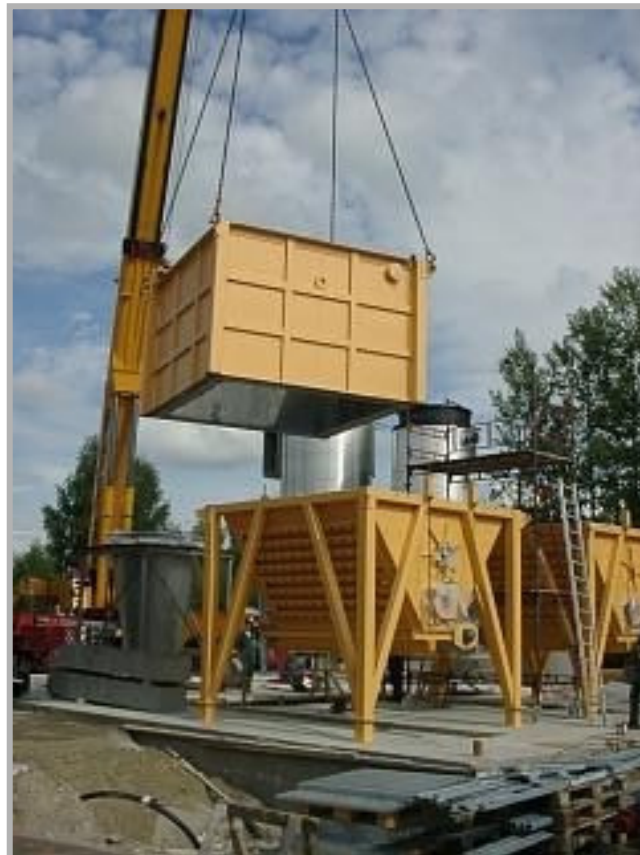
Figure 6 Primary chamber KENTEC ENERGY
