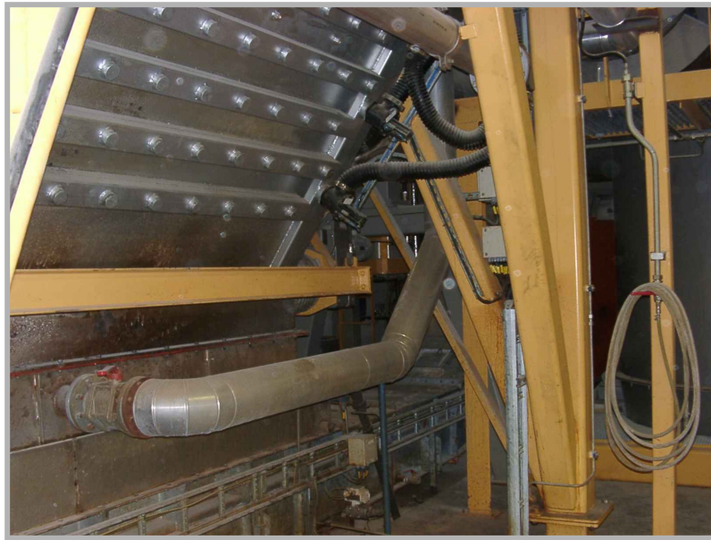
Figure 11 Primary air supply
