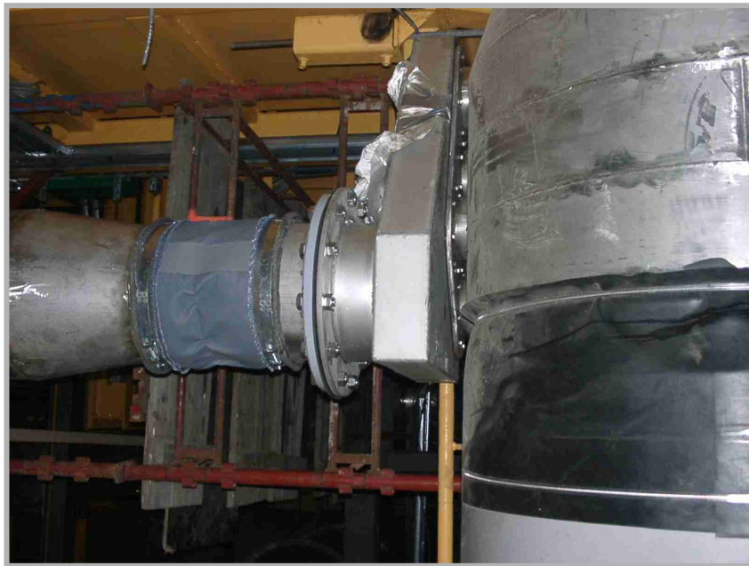
Figure 12 Secondary chamber manifold
